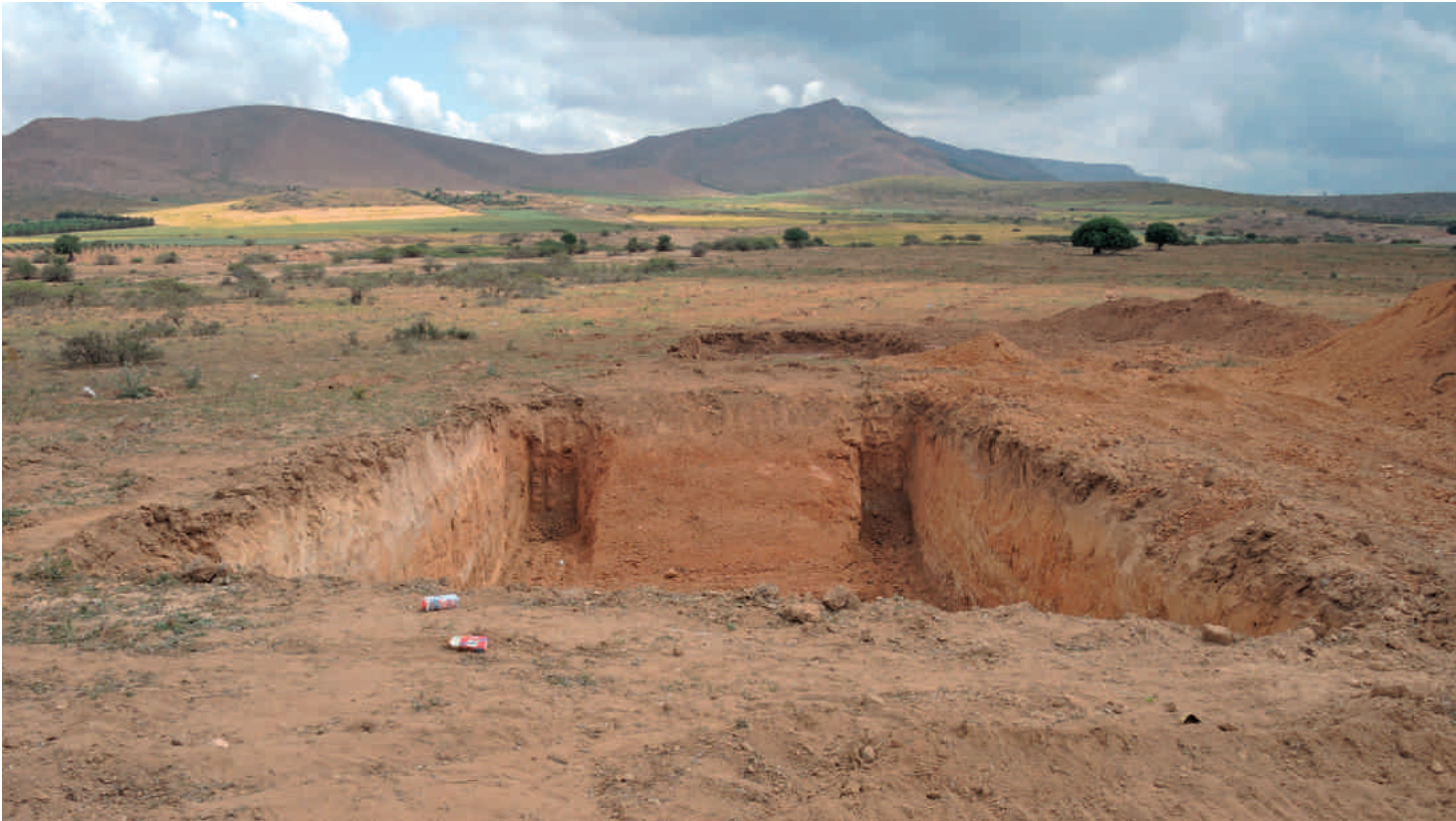
Preparatory work on a purification plant in the Region of L'Oriental, Kingdom of Morocco (2013).
